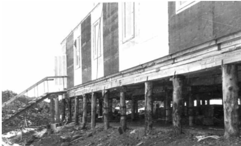
Fig. 5. Installation of quickly erected hostels for 60 persons with the pile wooden foundation and grillage in conditions of permafrost of the ground in the Far North
