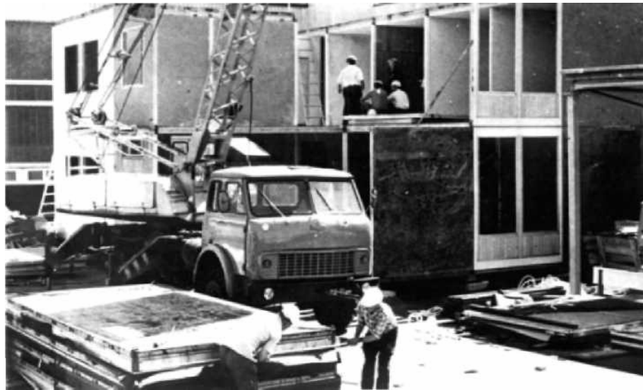
Fig. 8. Installation of two-storey apartment houses of the system "Module" near the city Stepanavan by the builders of the state cooperative enterprise "Lenooblagrostroy" (Stepanovan specialized building administration)
