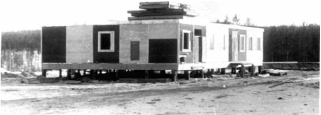
Fig. 6. Quickly erected kitchen - dining room assembled in conditions of the Far North at temperature up to -48^{\circ}\text{C} and speed of a wind up to 40\text{ m/s} without attraction of the building organizations
